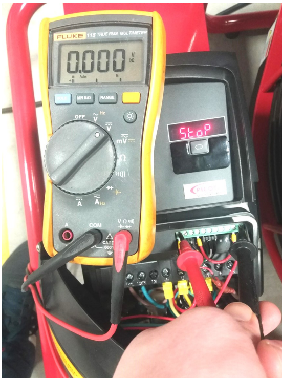
Emergency stop released
